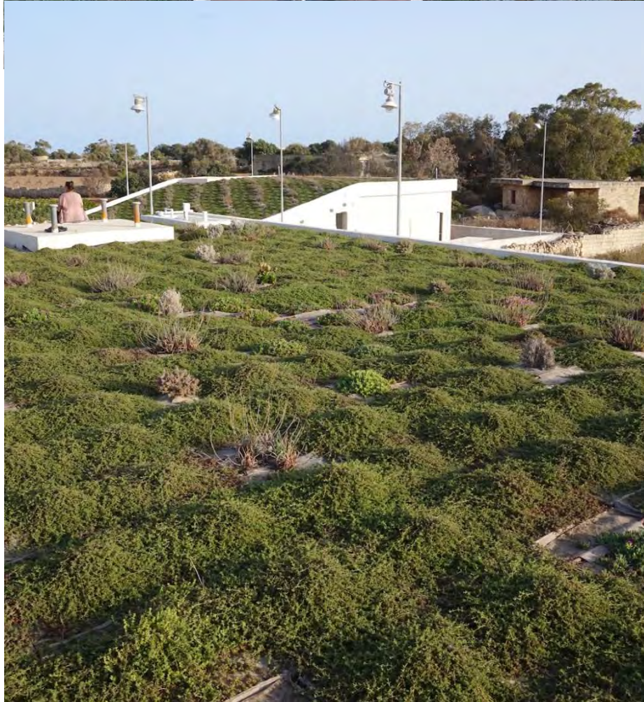
Figure 54: Green roof at Has-Saptan Enemed fuel depot facility (VIVACITY Ltd.)
